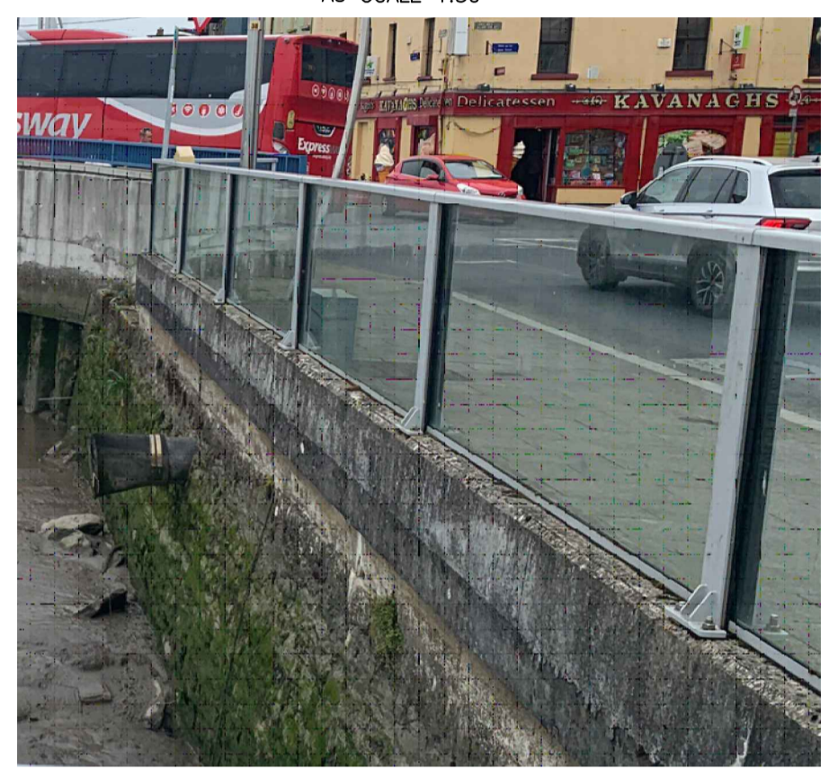
EXISTING GLAZED FLOOD DEFENCE WALL ON SOUTH-EAST QUAY (ADJACENT TO PROPOSED WORKS)
