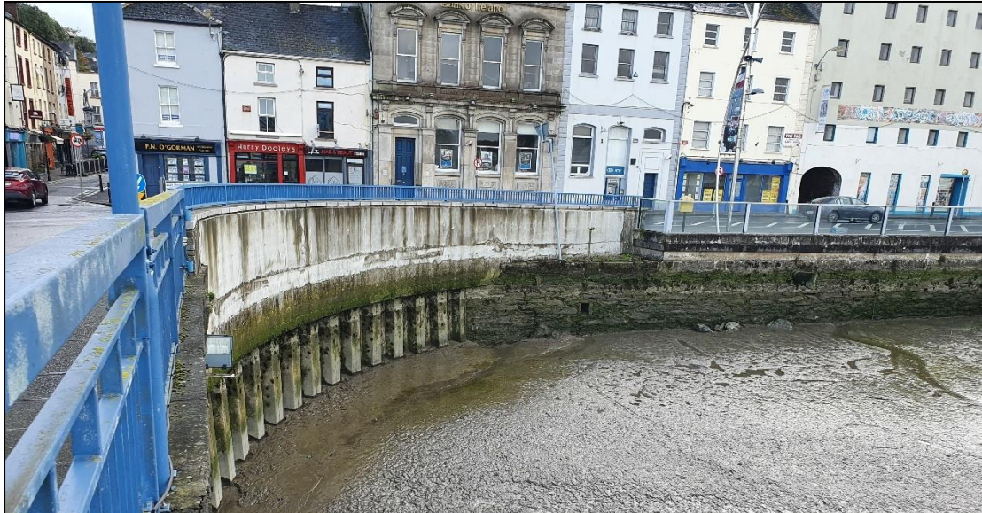
Plate 2-6 Masonry-clad reinforced concrete parapet wall developed as part of the New Ross Flood Alleviation Scheme (southeast corner)
