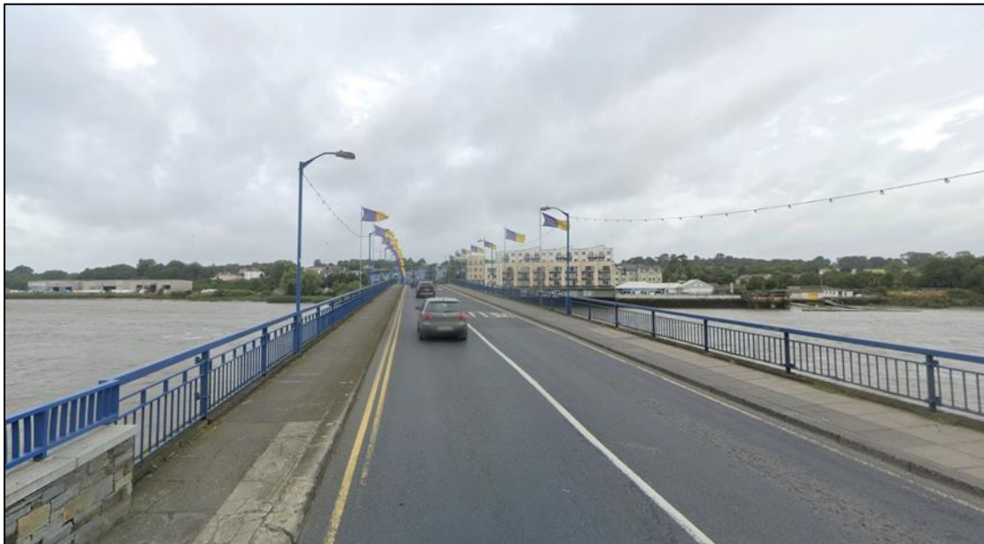
Plate 2.3 O'Hanrahan Bridge with view to the north-west. In the foreground are the existing road of the bridge and the narrow footpaths along the sides that are proposed to be widened as part of the development. The existing parapets are proposed to be replaced. © Google Street View
