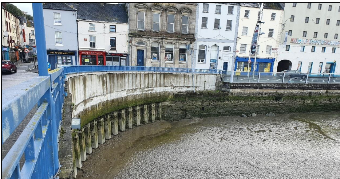
Plate 2.7 Masonry clad reinforced concrete parapet wall developed as part of the New Ross Flood Alleviation Scheme
