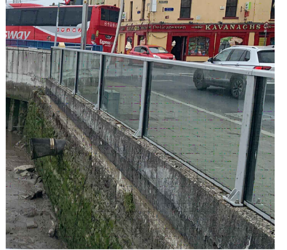
EXISTING GLAZED FLOOD DEFENCE WALL ON SOUTH-EAST QUAY (ADJACENT TO PROPOSED WORKS)
