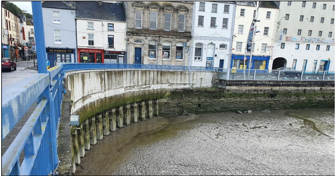
Plate 2.6 Masonry clad reinforced concrete parapet wall developed as part of the New Ross Flood Alleviation Scheme
